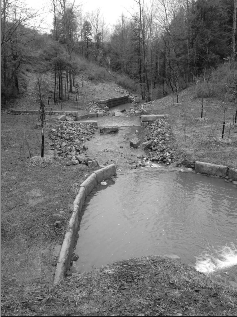
Figure 14 - Erosion Control Structures Installed on Erdman Brook. Shown are a series of pools and riffles. Looking downstream.
