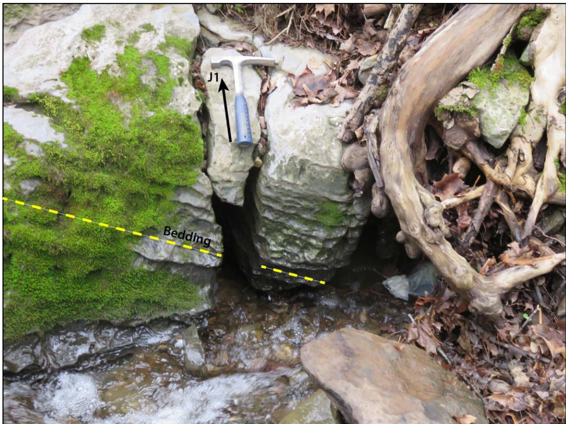
Figure 1-17. Swallow hole formed in J1 joints, located along the left stream bank and downstream from culvert 1. Water flow is from left to right, hammer for scale. Photo by R. Witte.
