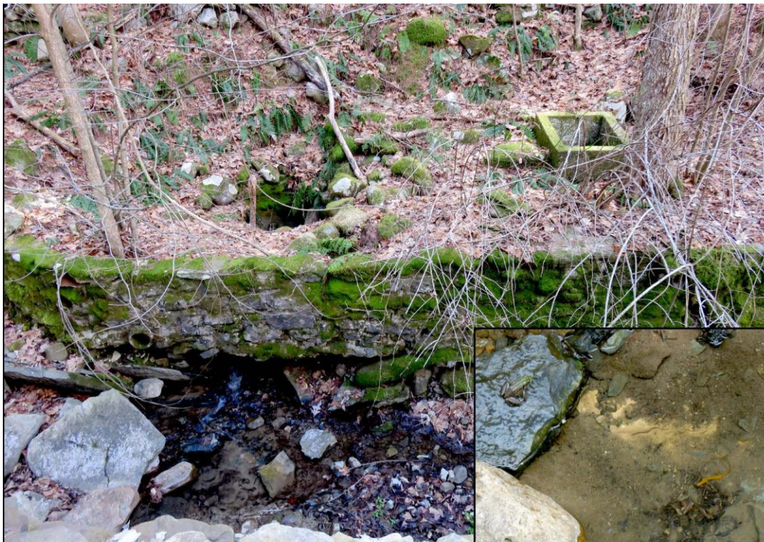
Figure 1-21. Small spring located just downstream from culvert 2. Over the years the low reservoir wall has been undercut resulting in the formation of a small sinkhole. Local denizens (inset photo) are the green-headed frog and orange long-tailed salamander, both common inhabitants of springs and seeps in karst areas. Spring photo by R. Witte and inset photo by Jon Inners.
