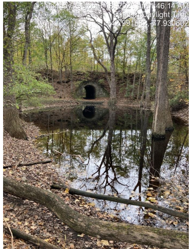
Figure 8. Water Table within the Mud Creek Swallet. Mud Creek flows into this feature through the railroad culvert.
